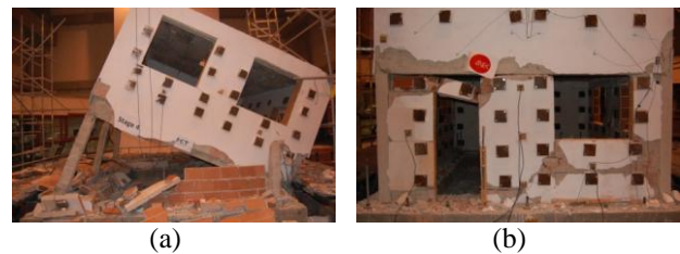
Figure 3: Observed damage at the end of the shaking table test: (a) model one; (b) model two
